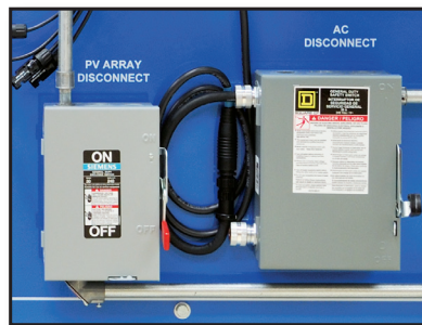
PV Array & AC Disconnects
